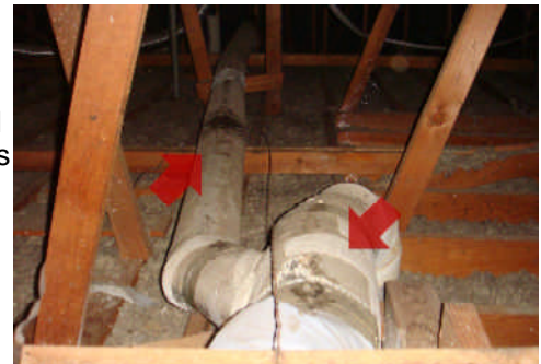
Soiled ducts from rodents. Health concern.
