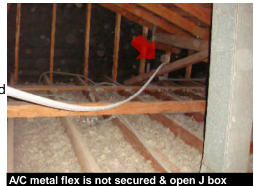
A/C metal flex is not secured & open J box
