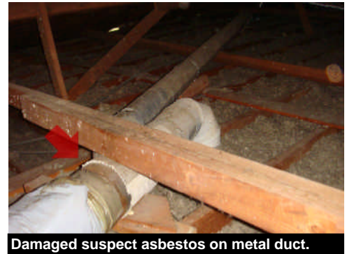
Damaged suspect asbestos on metal duct.
