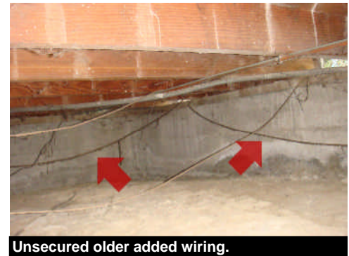
Unsecured older added wiring.
