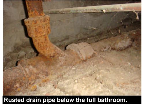
Rusted drain pipe below the full bathroom.
