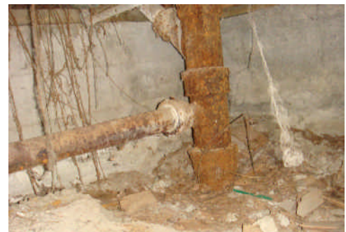
Rusted drain pipe below the 3/4 toilet.
