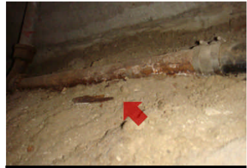
Metal is breaking off the cast iron pipe.
