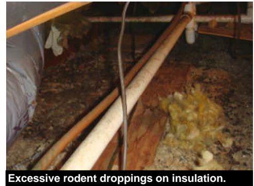
Excessive rodent droppings on insulation.
