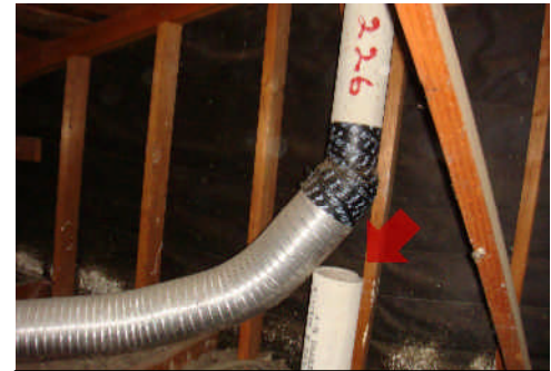
Broken in half transite pipe is asbestos.
