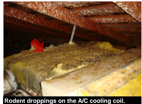
Rodent droppings on the A/C cooling coil.
