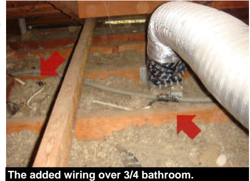
The added wiring over 3/4 bathroom.
