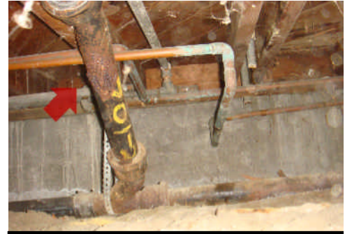
View below kitchen. Corroded cast iron.
