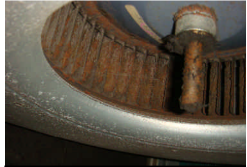
View of the soiled fan blades.
