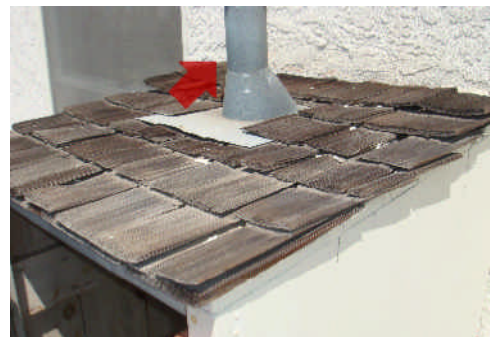
View also of the single wall vent flue.
