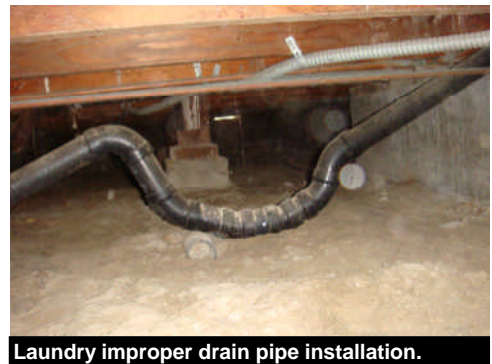
Laundry improper drain pipe installation.
