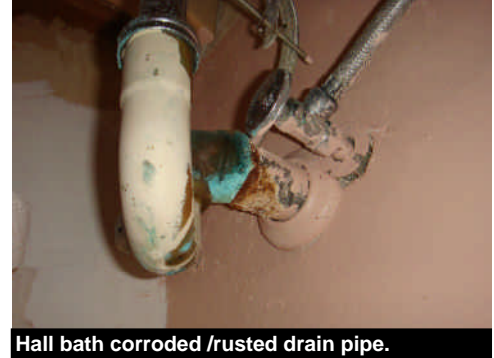
Hall bath corroded /rusted drain pipe.
